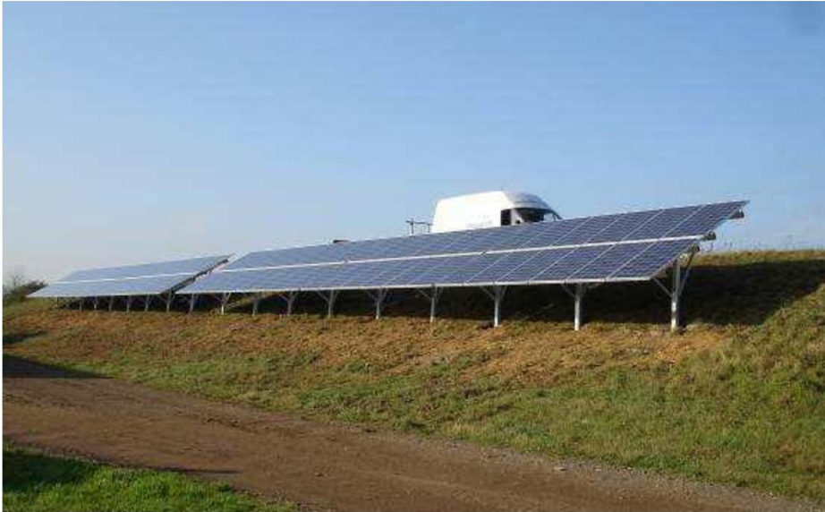
Photos of an installed 20kW ground mounted PV system.
